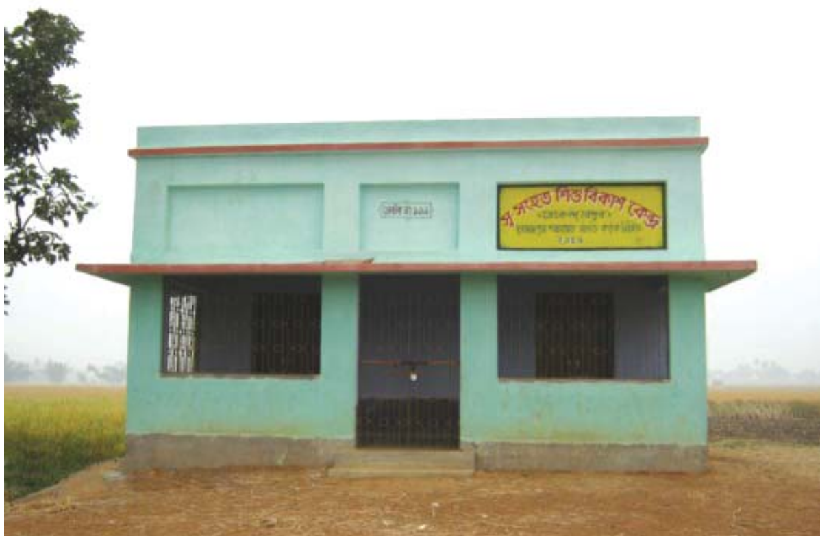
Public Health Centre constructed in Dubrajpur, Birbhum District (West Bengal) is in progress under MsDP Programme
